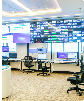
Capacity Management Center
